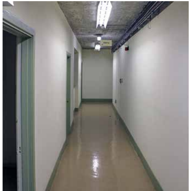
View of upper level corridor. In situ reinforced concrete roof is exposed at high level
